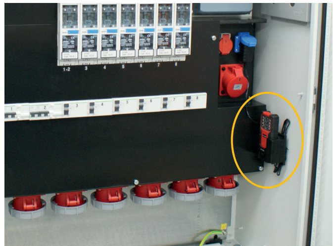
TorchLED Emergency in a construction site cabinet
